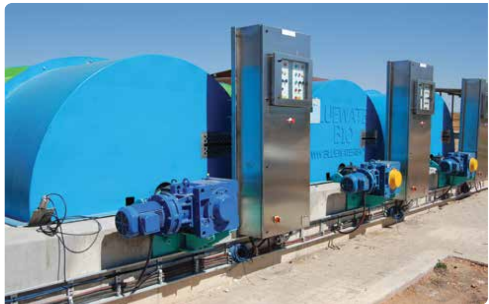
The SMART units at Hartbeesfontein WWTW
